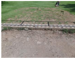
Absence of kerb ramp at level change
