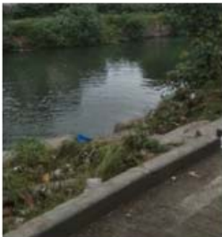
Barricates are broken around canal.
