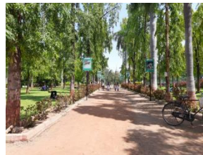
Improper road gradient along width
